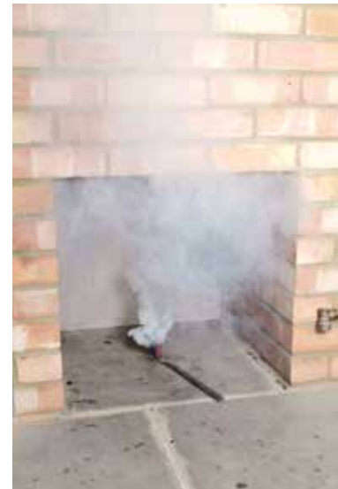
Figure 7.32 Flue flow test failed
