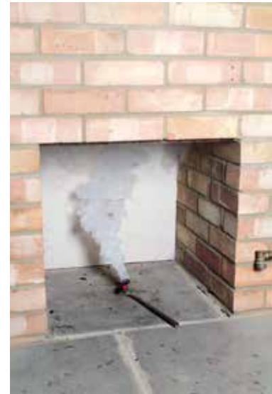
Figure 7.31 Flue flow test passed
