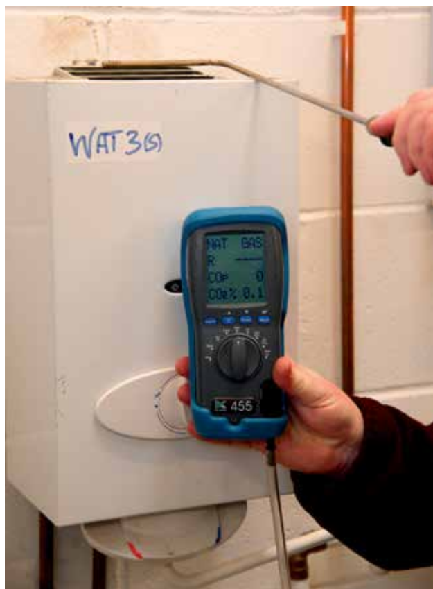
Figure 7.47 Angled sampling probe on a flueless water heater
